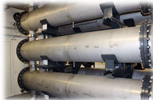
external heat exchanger
